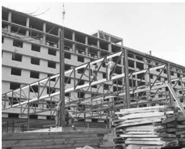
Oliver Hall in spring 1967, during its inaugural school year (top); during construction (middle); and on June 27, 2022, at the start of its demolition (bottom). By August’s end, the residence hall—named for KU’s first chancellor, R.W. Oliver—was no more.
